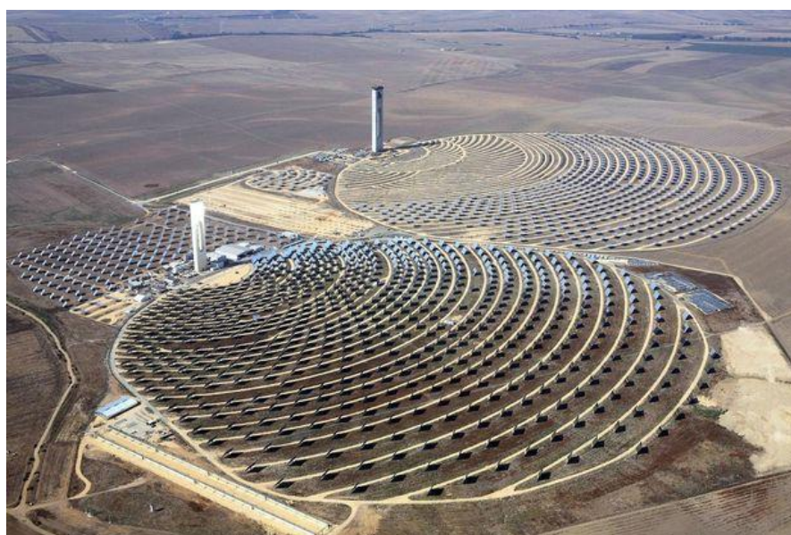
Figure 2 - CSP complex (World Bank image): Noor 1 (Left), Noor 2 & 3 (Right) to be completed in 2017 & 2018.
